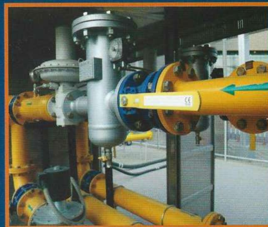
Pressure Reducing Station
